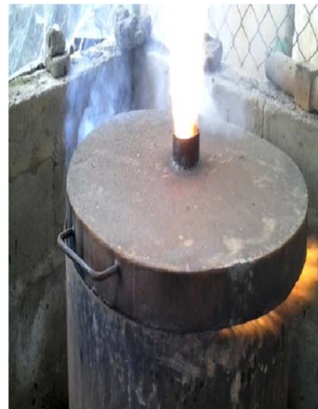
Figure 6. Chimney for keeping pressure balance.
