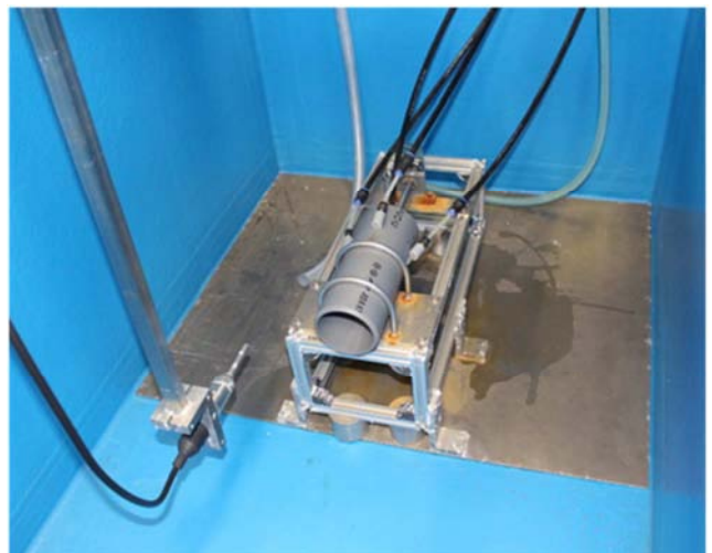
(b) Installed jet pump.
